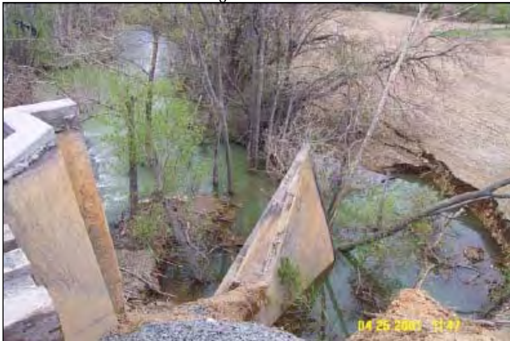
Figure 4.3.9-6. Norfolk Southern Railroad Bridge Wingwall Sinking into a Water-filled Sinkhole along Bushkill Creek
