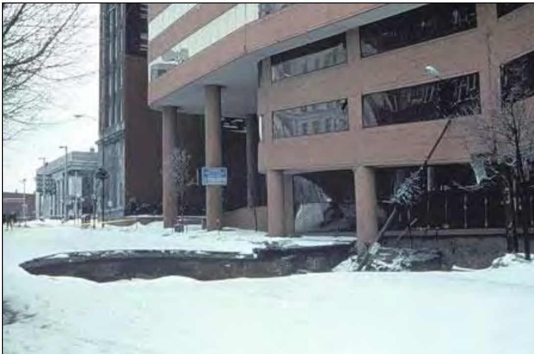
Figure 4.3.9-7: Sinkhole at Corporate Plaza Building in the City of Allentown, Lehigh County, PA in February, 1994
